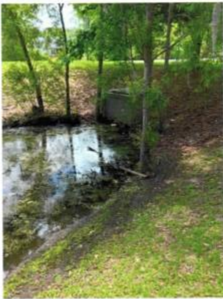
Debris blocking outfall structure
