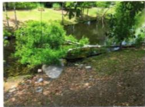
trees blocking inlets/ refresh rip rap
